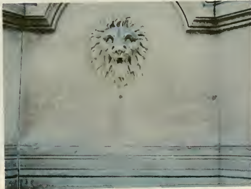
Figure 28: Evidence of inappropriately removed graffiti from pedestal
